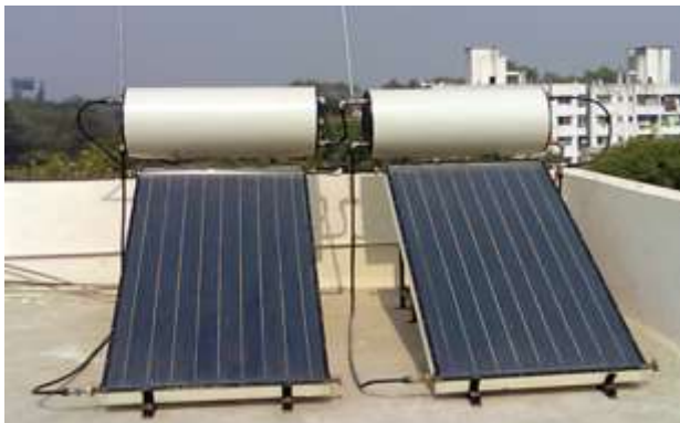
Solar Water Heaters
