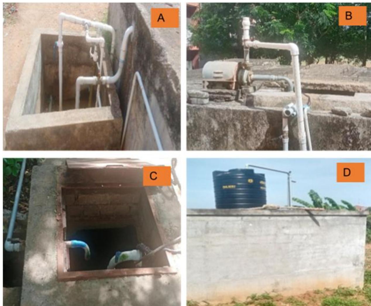
Figure 4: Wastewater treatment facilities at Nehru Arts and Science College
