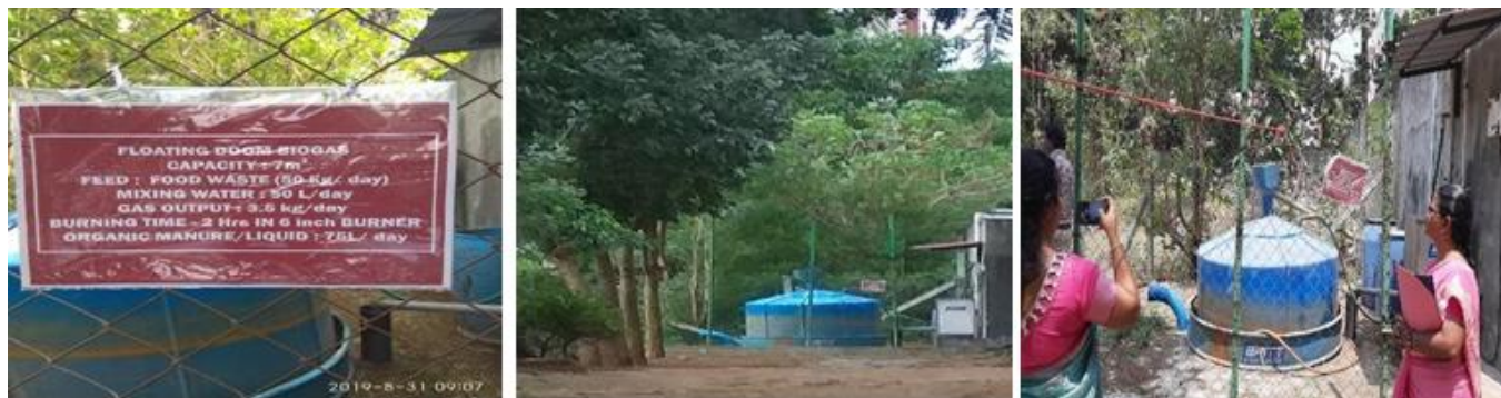
Figure 2: Biogas facilities at Nehru Arts and Science College Vermicompost / Organic manure production
