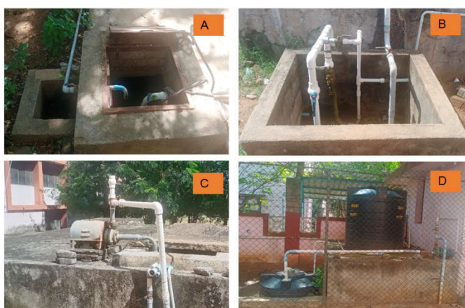
Fig 1 Wastewater recycling facility installed at Nehru Arts and Science College campus
